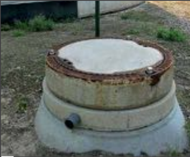
The condensate pit is a place where your personal safety may be at stake. The explosion label is somewhat misleading because the danger comes from the concentration of carbon dioxide down in the pit. There is acute suffocation hazard! Enter the pit only well secured and with personal protection equipment by climbing down a ladder.
