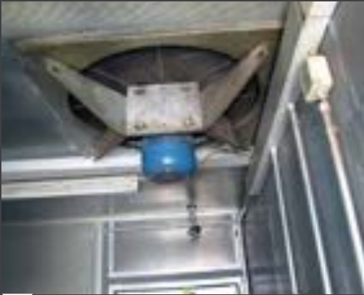
The ventilation of the cogeneration container is very important to prevent overheating and fire.
