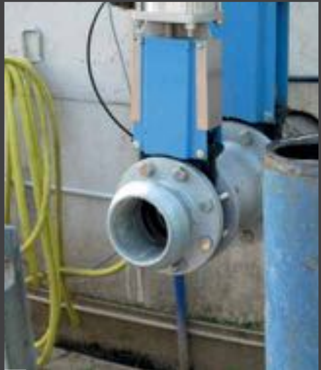
The air from the blower supports the foil roof. The blower will give good and lasting service provided it is inspected and cleaned regularly.
