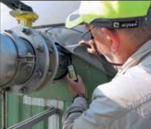
The portholes should be checked during the daily inspection tour of the plant. The owner will have a look in the digester anyhow – then why not look at the porthole and the area around it as well?
