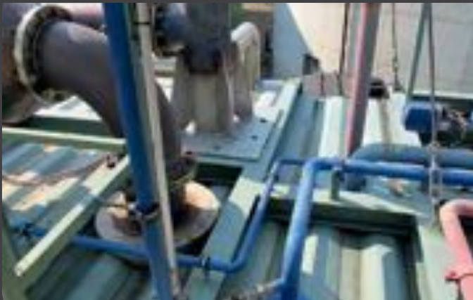
Proper bolting of pipe connections installed on the roof of the cogeneration container is important.
