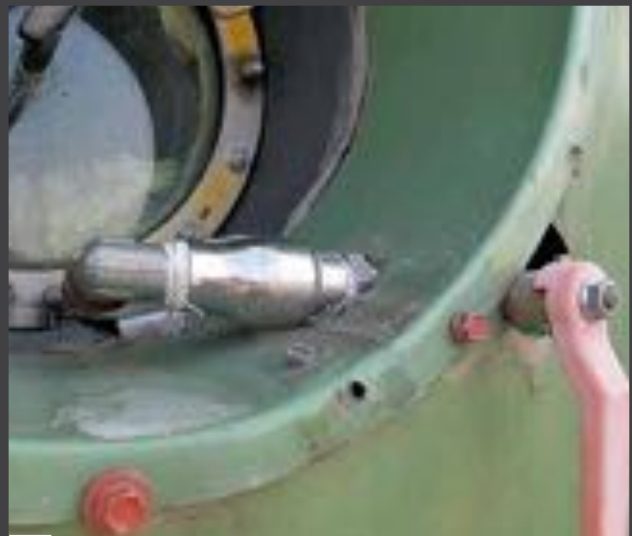
Pipe leadthroughs and connections are potential sources of leaks. Gas losses due to leaks can add up to a total of 1,000.00 euro a year in a 500 kW plant. The investment in a gas meter will be recovered quickly.
