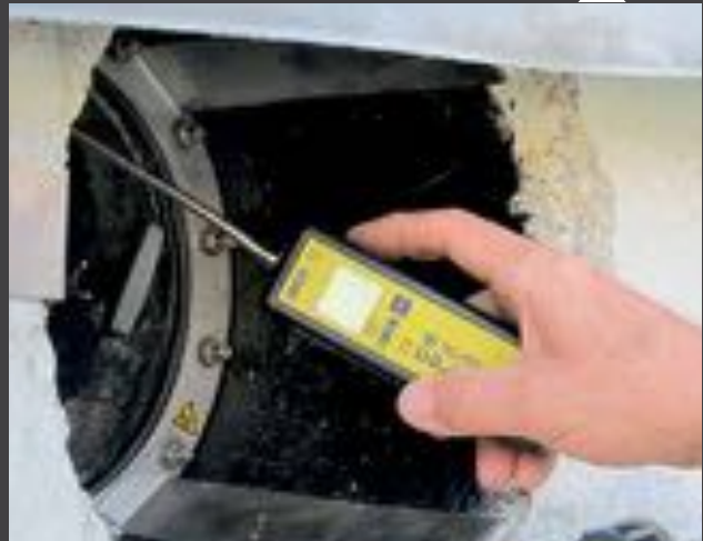
The point at which the agitator enters the digester should be inspected for leaks. The ventilation should also not be bypassed but checked.
