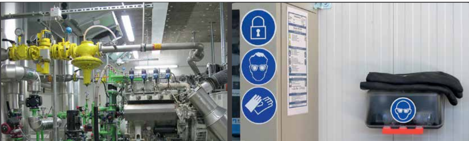
Good lighting of the cogeneration room improves safety and makes work easier Personnel protection equipment should be handy and marked.
