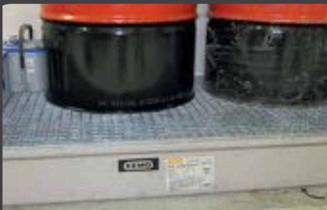
A catch basin must be available where water-polluting fluids are handled.
