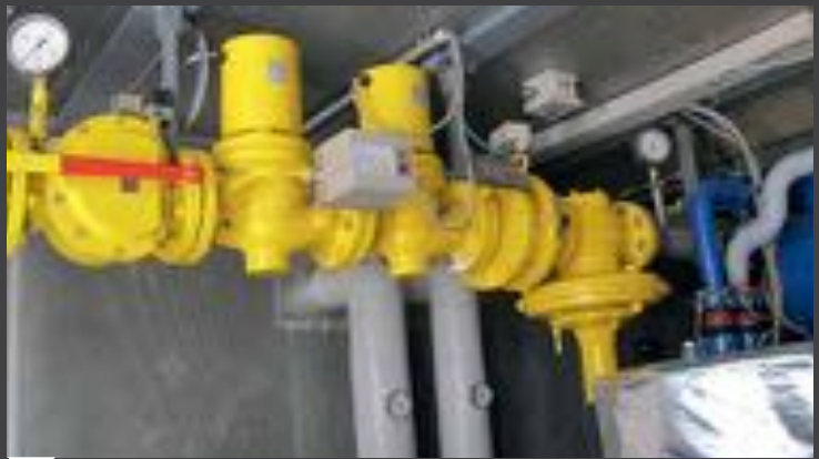
The pipelines with gas in the cogeneration room must be inspected. A gas detector is obligatory here.
