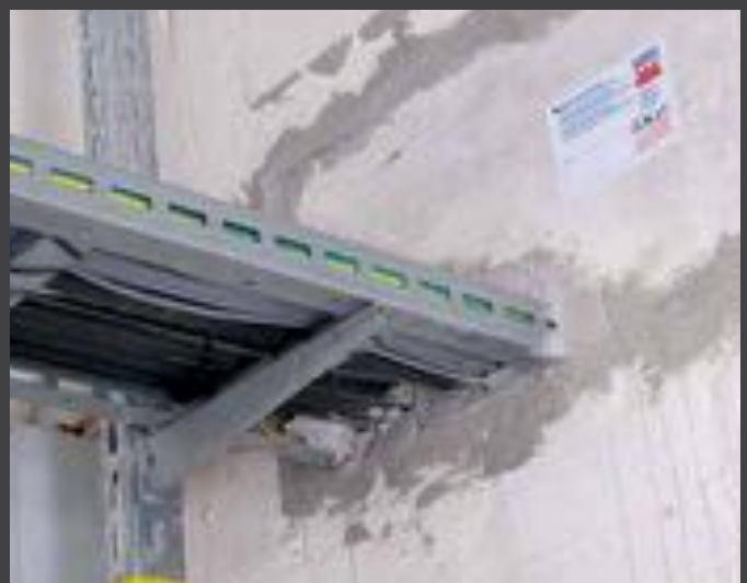
The fire protection function must be restored where a hole is cut in a fire wall. A badge provides the required information. An electric check must be made every three years. This is a one-and-a-half day job for a trained electrician.
