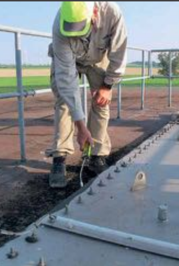
If covers are installed on the digester roof, the seals need a close look. A gas leak tester will provide reassuring results.
