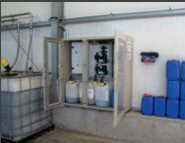
The storage of trace elements and their dosing are exemplary in this plant. Computer programmed dosing minimises the hazard for the operator.
