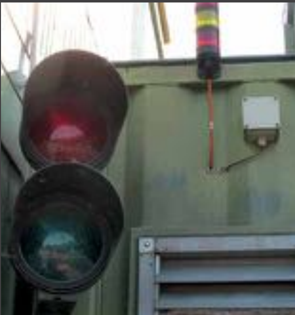
Visual and audible warnings are required to signal the state of the plant to rescue personnel on their arrival. Suitable rescue measures can be taken more quickly.
