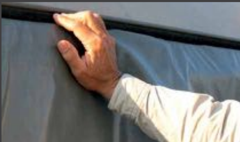
The cords on the foil roof are exposed to particular wear and tear due to wind and weather, and should therefore be inspected regularly.
