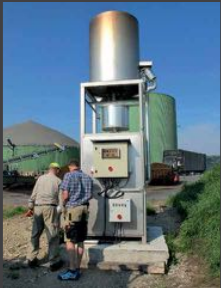
The biogas flare should be state of the art and always ready for operation.
