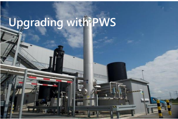
Biogas upgrading plant (based on Pressurized water scrubbing technology): processing 550 Nm 3 of biogas per hour for distribution into the Dutch national gas grid.
