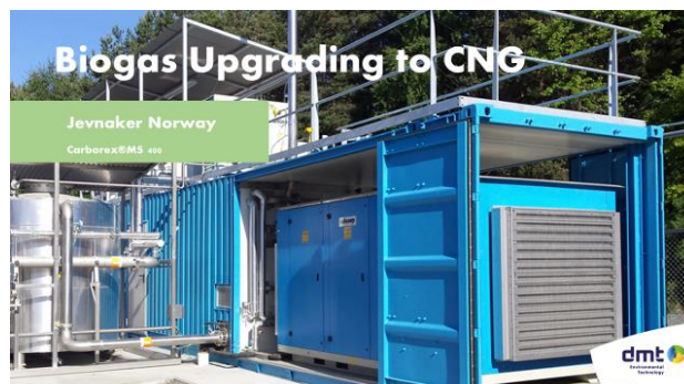
Biogas upgrading plant – Carborex MS (based on Membrane separation): processing 400 Nm 3 of biogas per hour to CNG (on courtesy of DMT).
